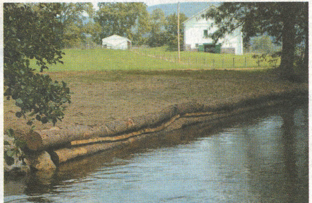
Above, a 100-foot mudsill enhances habitat and helps stabilize the stream bank. Above right, spectators during the Sheep Farm Project.
