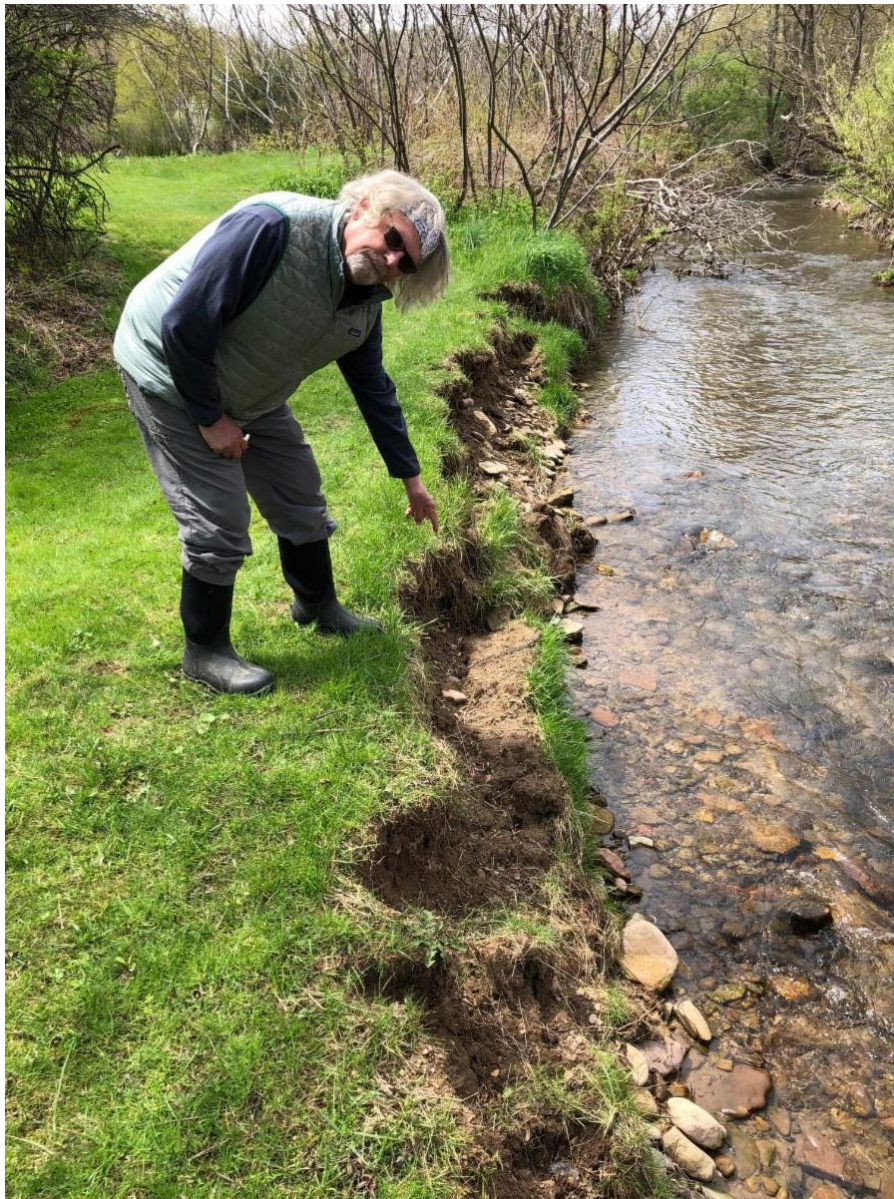
Example of bank erosion at Sparrow Run
